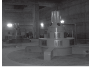
Büyükbahçe HES 2x6,050 MWm 2x5,850 MWe
